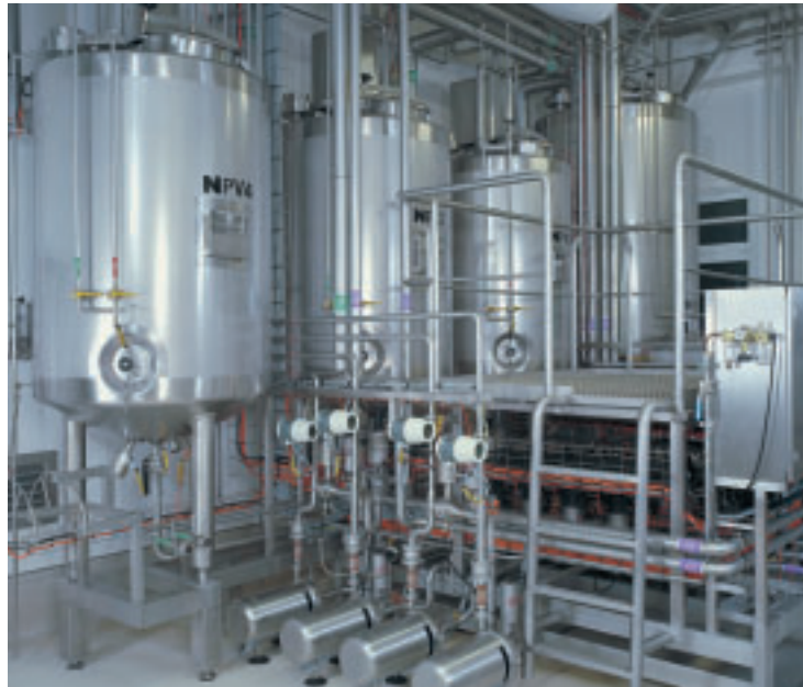
Automated, recipe-conducted mixing plant
